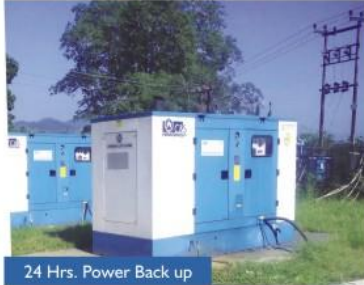
24 Hrs. Power Back up
